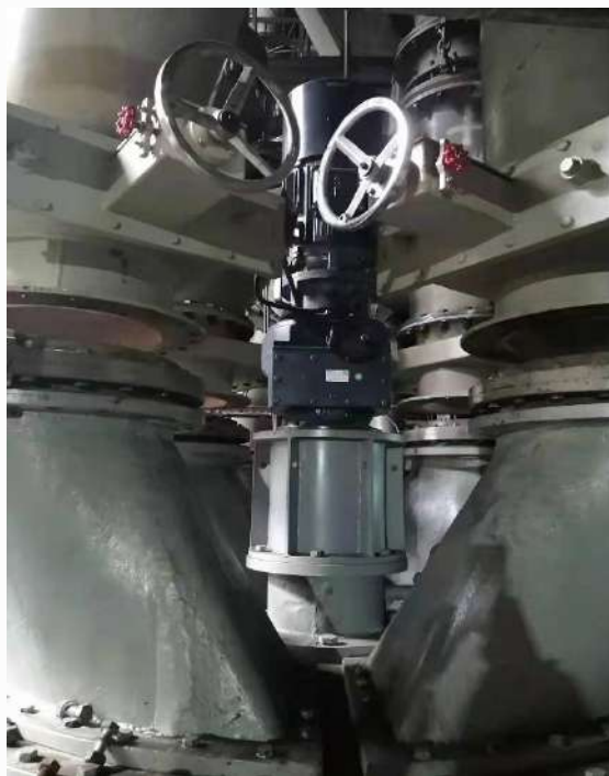
Taiwan Peace Power Plant
