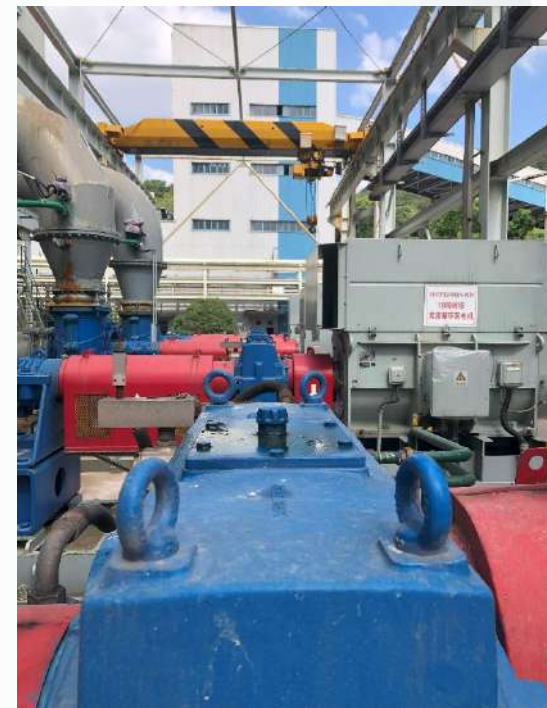
Ninghai Power Plant Desulfurization pump
